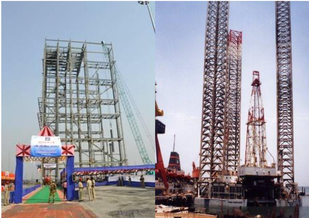
Boiler drum lifting unit being built at Kanti Thermal Power Plant in Muzaffarpur.
